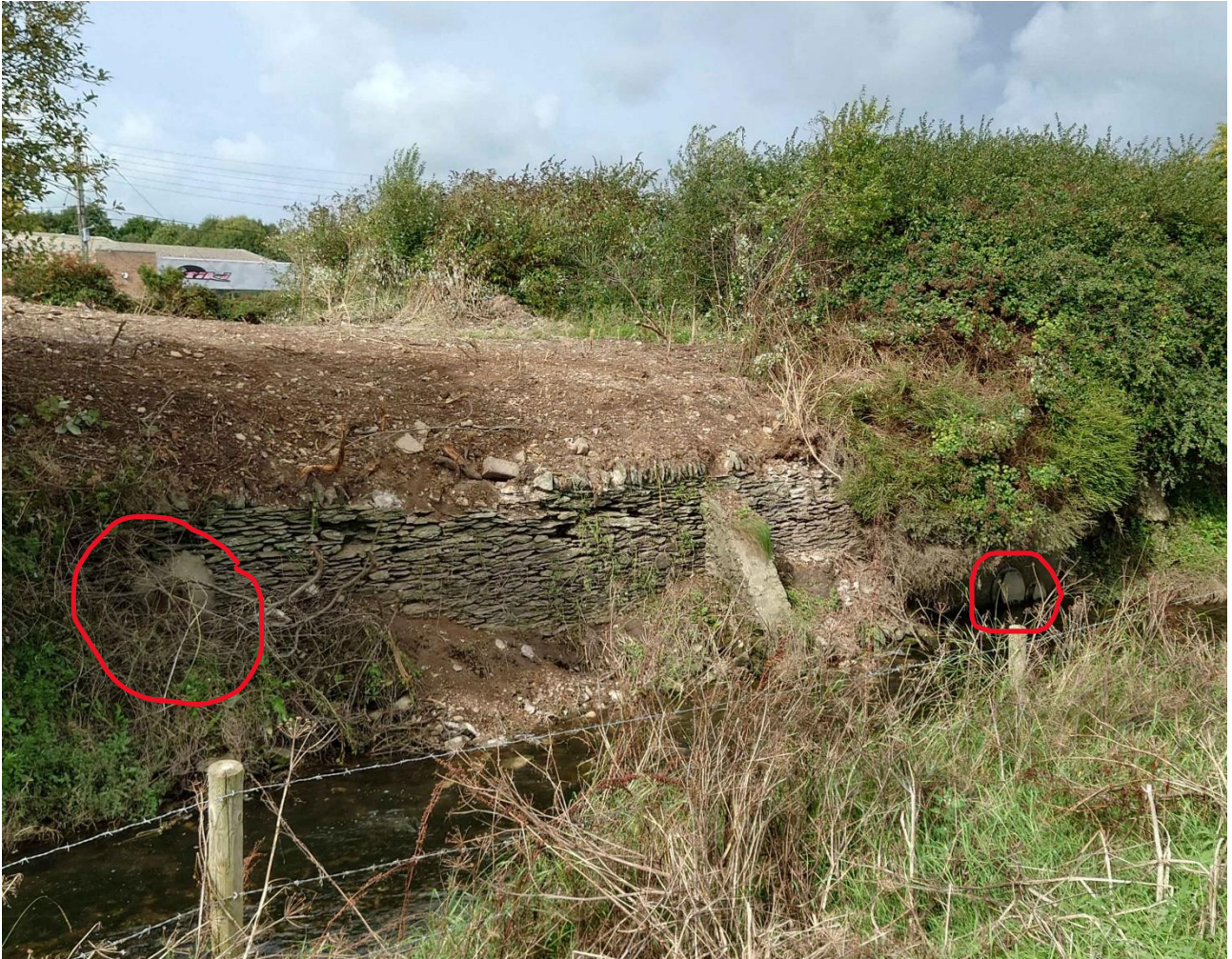
Photo 2 – The two outflow points above Knowl Water in wall in state of poor repair
