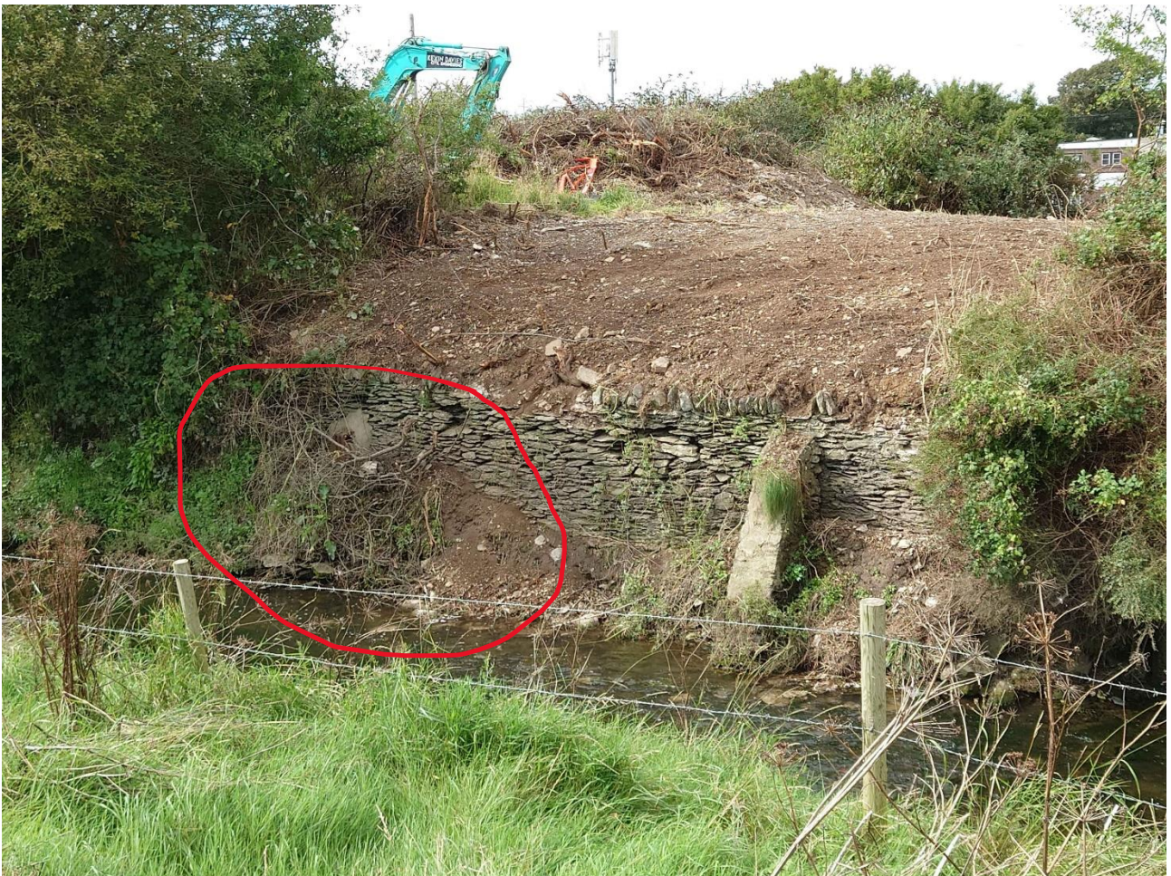
Photo 1 – blocked outflow pipe
